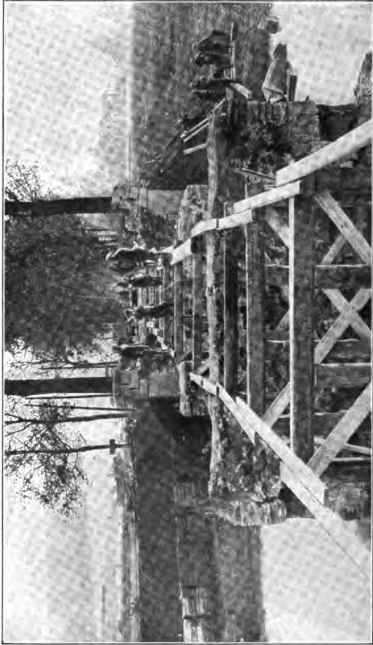
AMERICAN ENGINEERS REPLACING A BRIDGE AT GRAND PRÉ, THREE TIMES DESTROYED BY SHELLS
